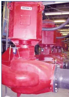
Enwave District Cooling Facility, Toronto, Canada.
