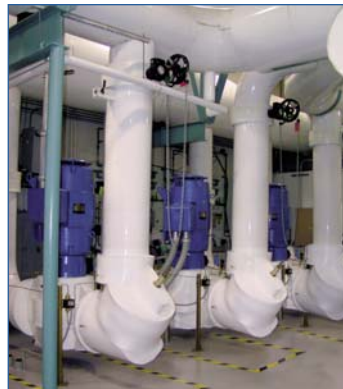
District Cooling Project, Phoenix, U.S.A.
